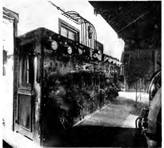
FIG. 4.—VIEW OF SWITCHBOARD.
